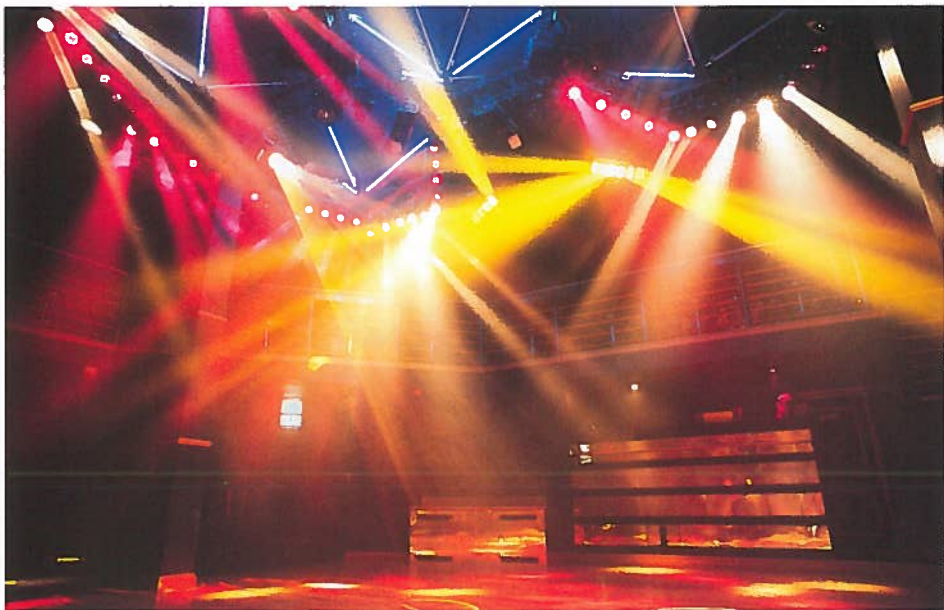
Above, the main dance floor at Xtreme and below right, the control set-up with Light Processor's Integrator desk taking the lead role. Photos: Graham Goldwater
