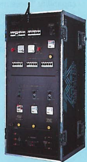
Mains Distribution System
