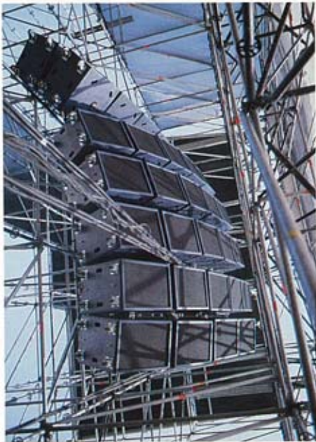
The main flow Flashlight system within the PA tower.
