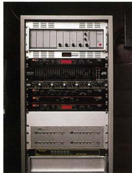
A typical 'orbit' slave amp cabinet installed in the risers.
