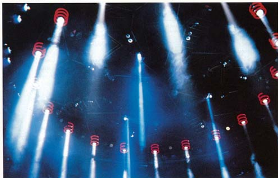
ACLs mounted on the ceiling inside red neon sculptures. Each of the 54 red rings is on a separate control circuit, providing many different chase possibilities.
