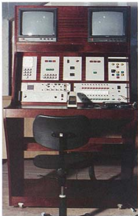
The stage manager's room complete with Clear-Com intercom facilities.
