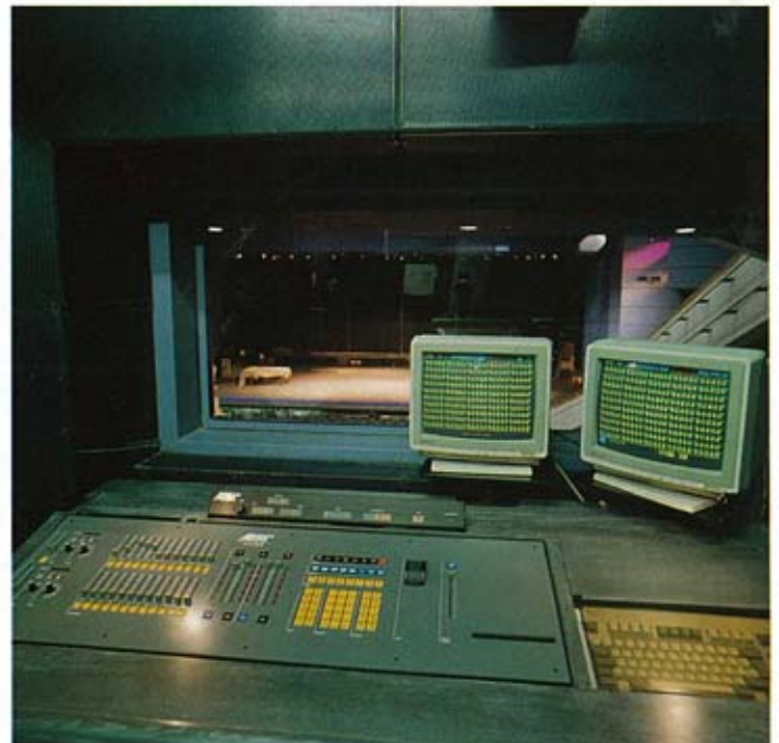
Arri Imagine 500 in the Hall One control room.
