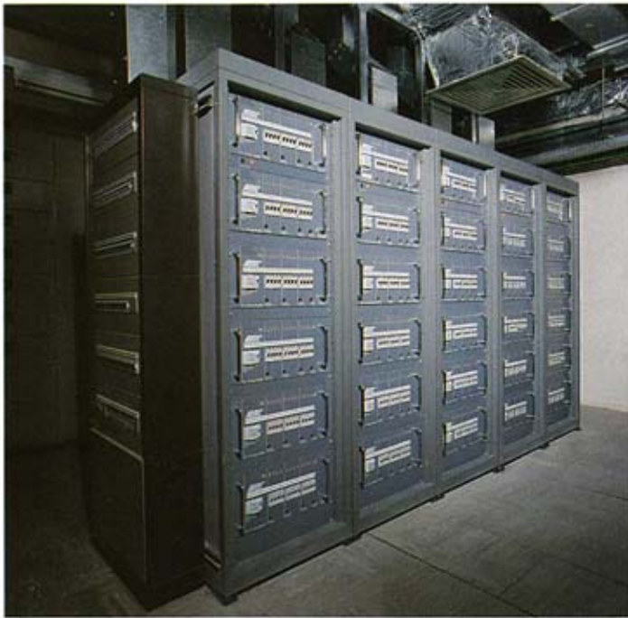
Arri dimmer racks in the South dimmer room.
