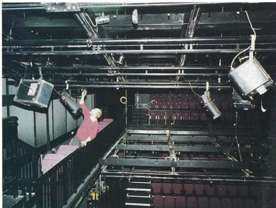
Old Fire Station Studio Theatre: an overview of lowered rigging system.
