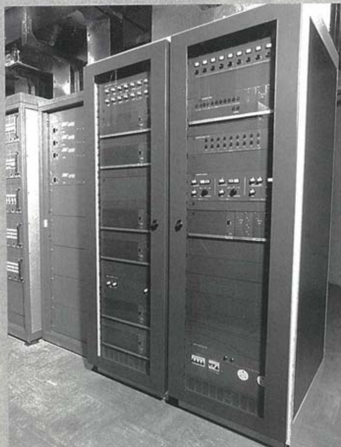
Dimmer room at the ICC, Birmingham with Glantre houselight control racks in the foreground.
