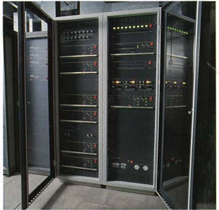
Glantre control racks, South dimmer room.
