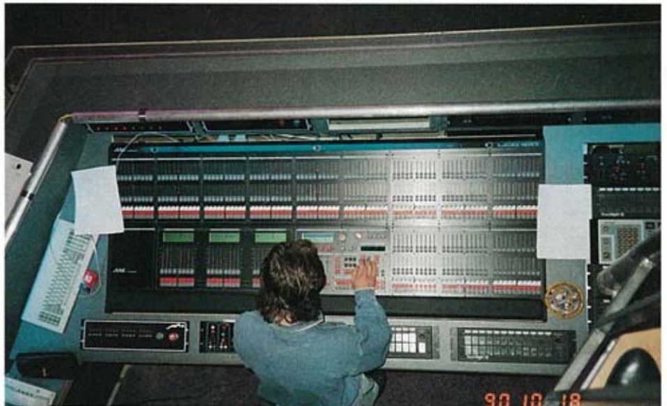
This LCD120 desk was installed at 'M' discotheque in Cologne in October 1990.
