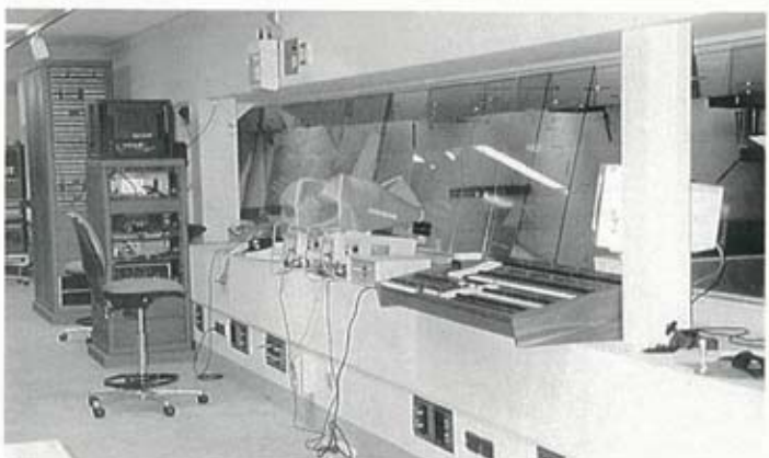
The control room for the John Batman Hall with Strand's Lightboard M in the foreground.
