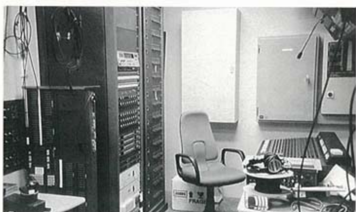
The modular amplifier rack room, with mobile Yamaha audio console in the Bellarine Banquet Hall.
