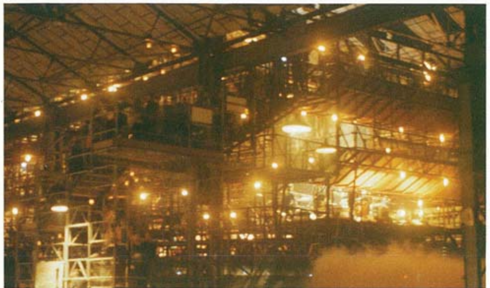
Looking from behind the constructed stage (right) along the length of the warehouse.
