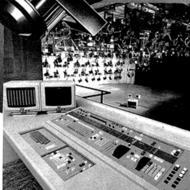
Lighting rig in Studio 1 at VTO-Medienzentrum Studio Complex, Hannover, showing Galaxy Studio remote control (on studio floor) & Galaxy 2 lighting console (in vision control room)
