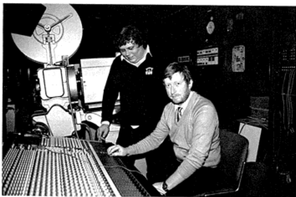
Steve Easy, stage director of the Orchard Theatre Dartford (left) and Ken Priddy of Luff Light & Sound with the new Allen & Heath Sabre sound consoles Luff's have just supplied and installed at the venue.
