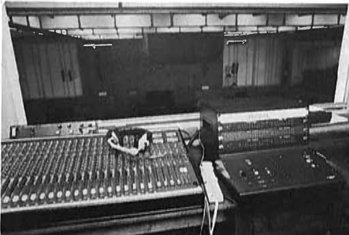
Sound control with cluster control to the right.
