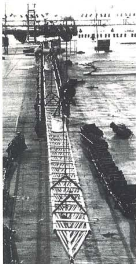
"The longest truss in the world" - for the 1987 Royal Tournament at Earls Court. The event is an annual four-in-hand between producer Major Michael Parker, lighting designer Robert Orno, Theatre Projects and The Unusual Rigging Company Limited.
