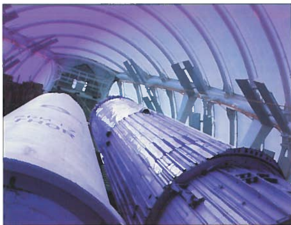
Above, the 42m tall Rocket Tower with above right, Robin Elias, project leader at Unusual Rigging, working on its installation
