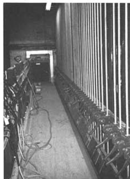
The new operator gallery with re-positioned rope locks - originally at stage level.
