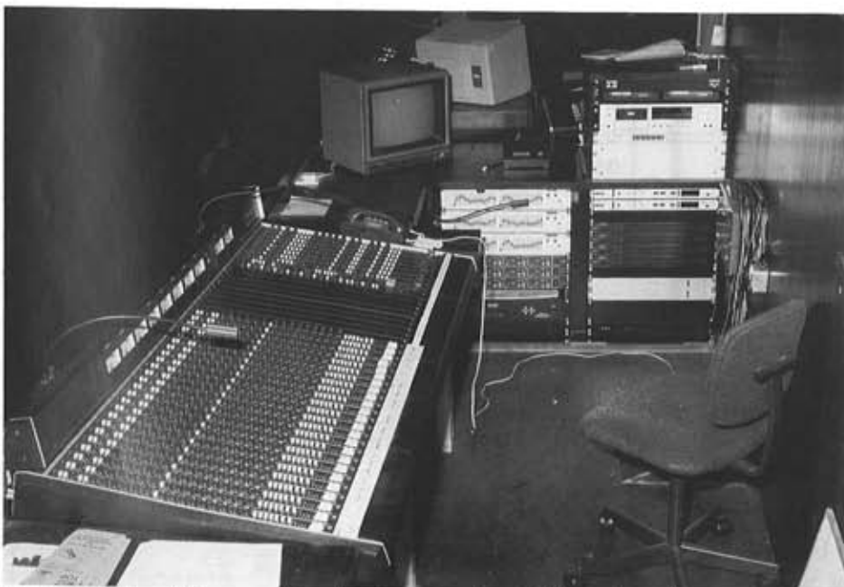
Compact sound control area provides adequate space with no sightline obstruction.
