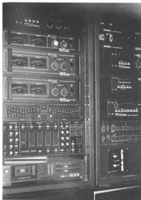
Operator's corner at the 'Black Hole'.
