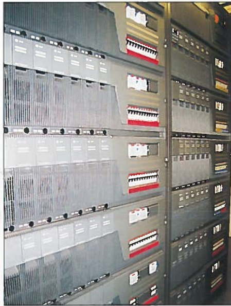
Strand EC90 modular racks dominate the remote dimmer room.
