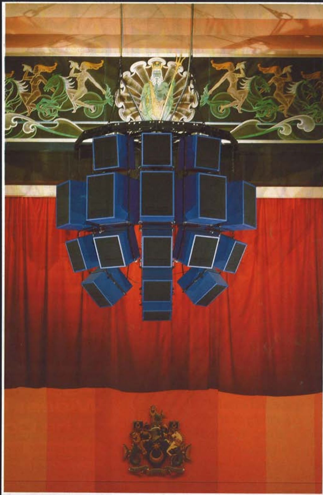
Turbosound's recently installed TSE system at the Guildhall Portsmouth (see second feature on cluster sound systems in this issue)
