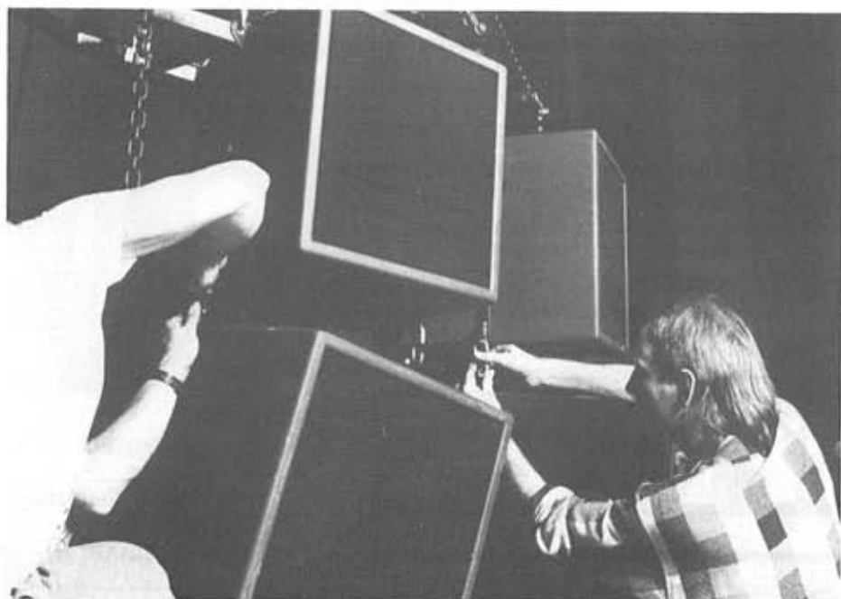
David Bearman (left) and John Newsham working on the Portsmouth Turbosound installation.
