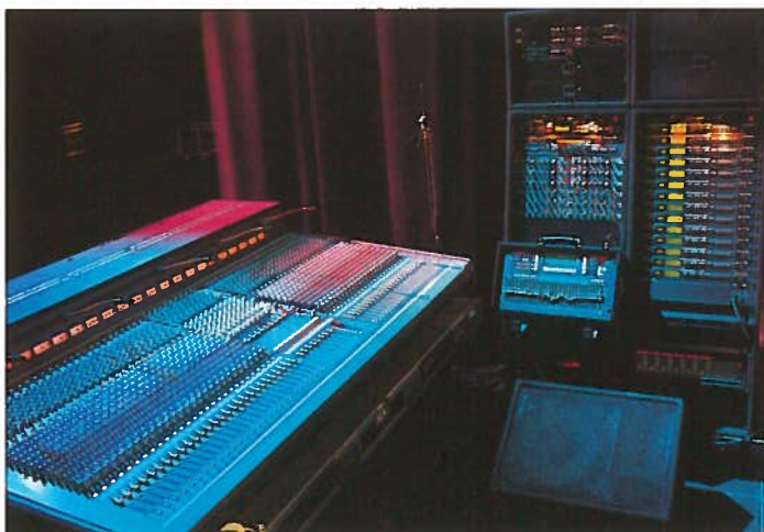
The Yamaha PM4000 at the front-of-house position in the main hall.
