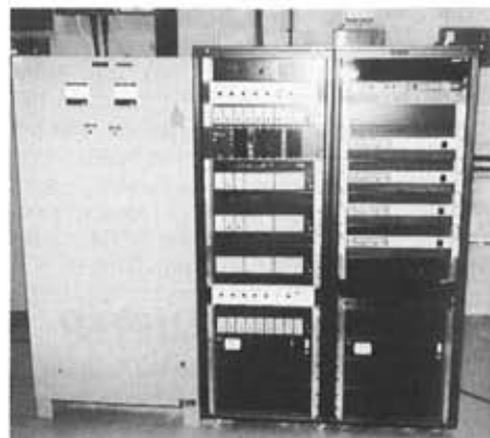
Slough Ice Arena - amplifiers on right, processors in centre, and stand-by batteries on the left.
