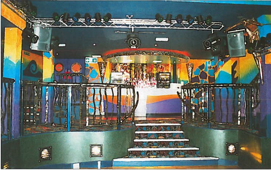
The Martin Audio speakers installed at The Lido in Truro, Cornwall.
