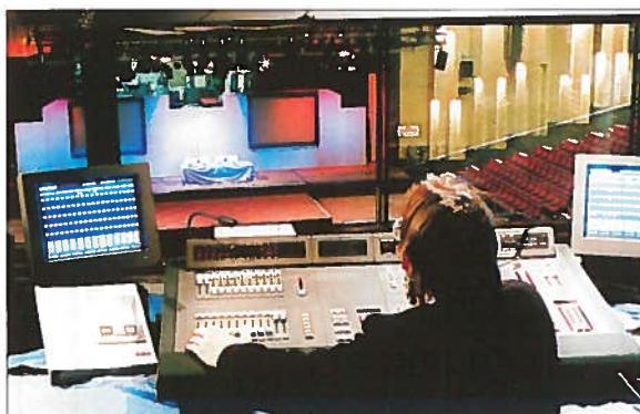
The stage as seen from the control room.
