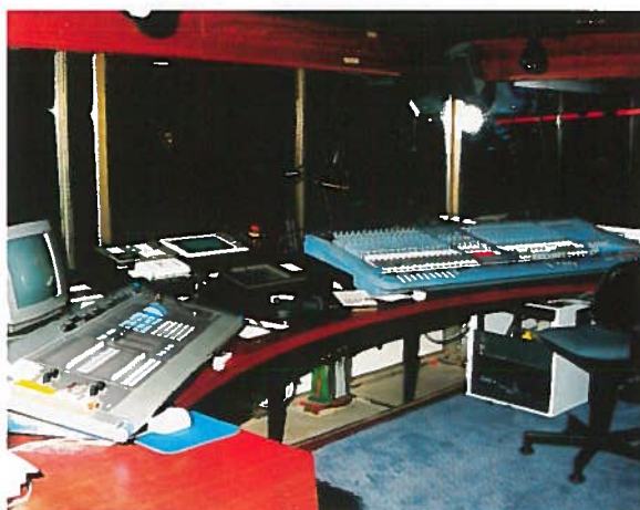
The main control room for Theatre Royal.
