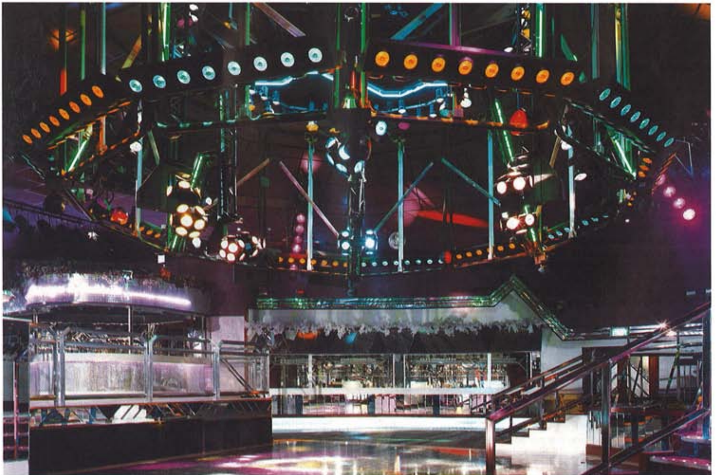
Custom-built light bars at Mr. Smith's in Warrington are moved by means of Origa pneumatic cylinders, and controlled by a purpose-built control system. The complete scheme was designed by Graham Barron for Satel, with rigging by Astralloy, lifting by Dagar, sound by Abacus, lighting by Satel and installation by Action Light. Current projects being worked on by Graham Barron of Satel include The Quadrant at Bootle, and The Carlton in Liverpool.
