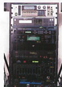
A rack of processing under the command of Theatre Sequencer.
