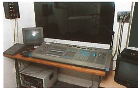
Coliseu: Arri Imagine 2 in lighting control room.
