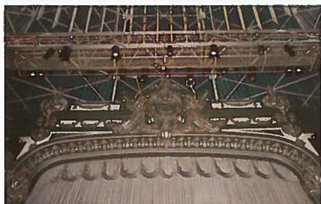
Juliat luminaires below auditorium catwalk.
